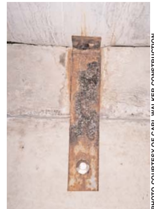
A corroded connection.
