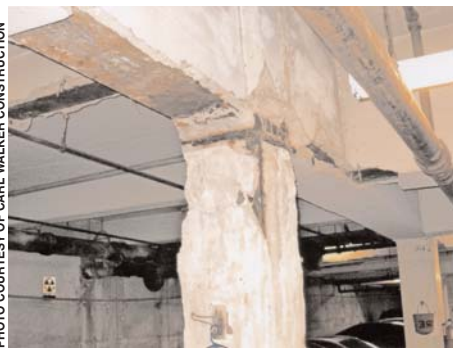
Column beam spalling.
