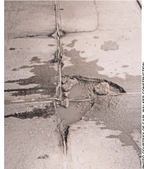
Floor demolition spall.
