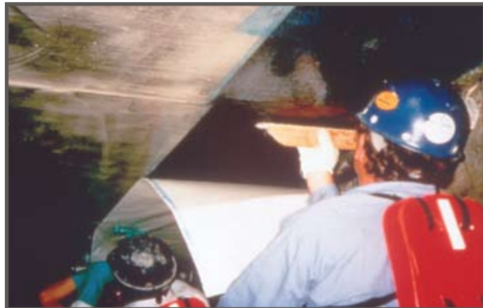
Overhead application at hospital to strengthen floor for high density filing system.
