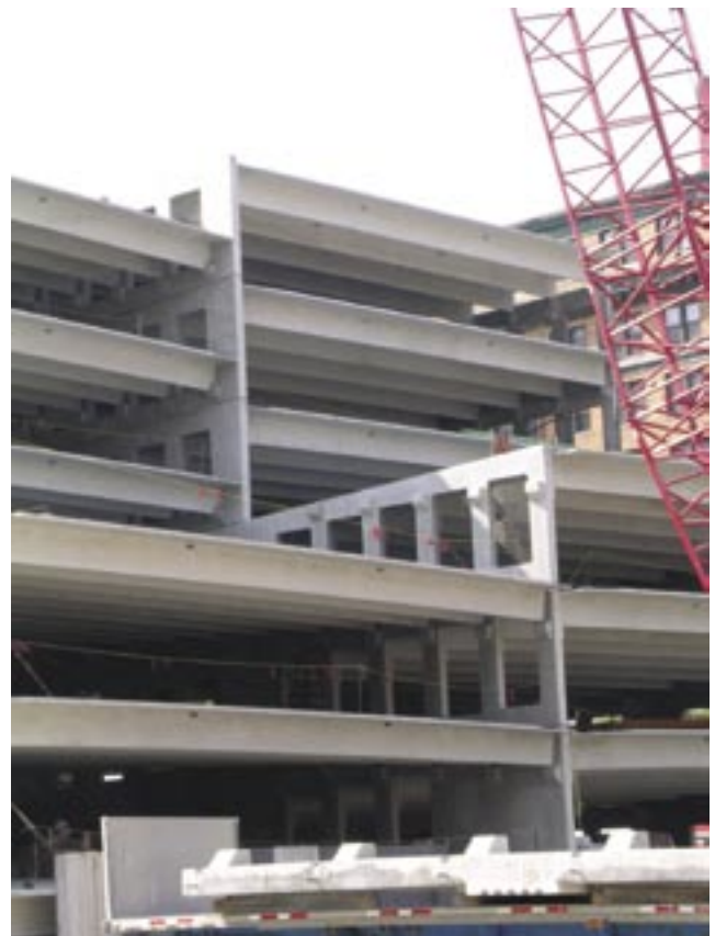
Fig. 1: A partially-completed precast concrete parking structure consisting of key components including columns, double tees, inverted tees, and shearwalls
