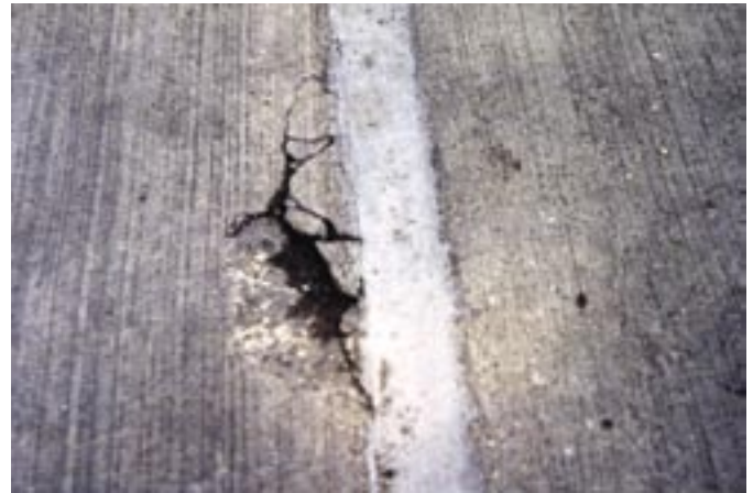
Fig. 3: Cracking and edge spalling behind the flange connections can occur if the joints are not properly detailed
